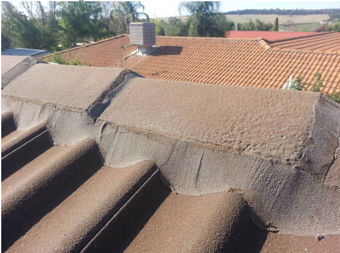
Photo 2: Example of hairline cracking to the pointing.
