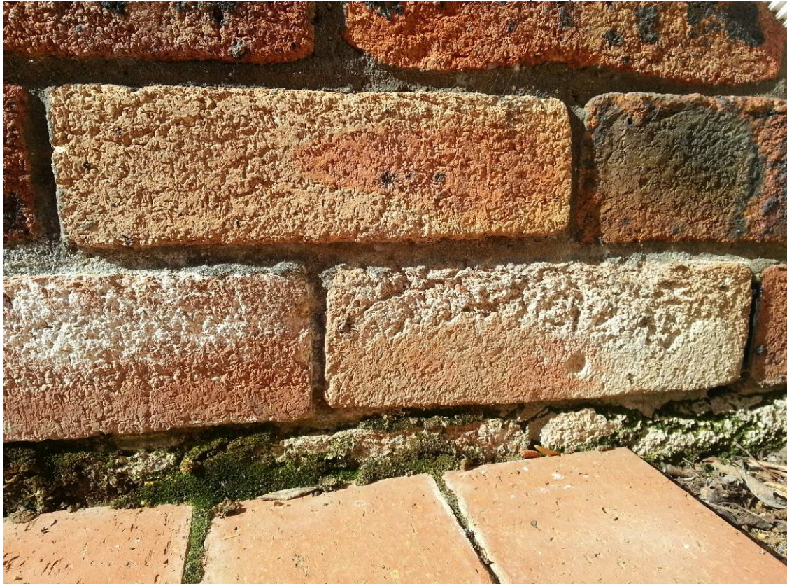
Photo 1: Minor fretting of the brickwork and efflorescence.
