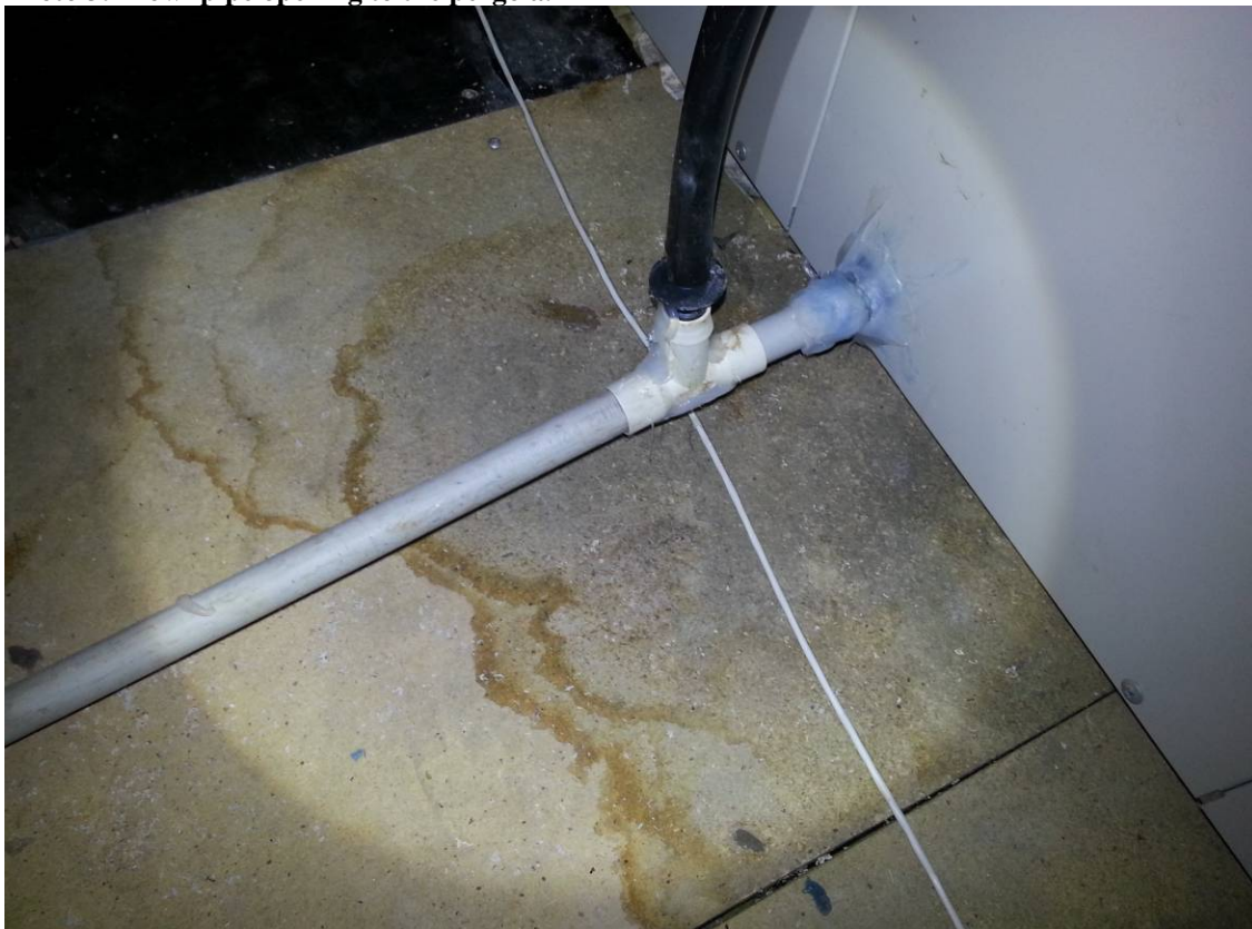
Photo 4: Water staining beneath water runoff line.
